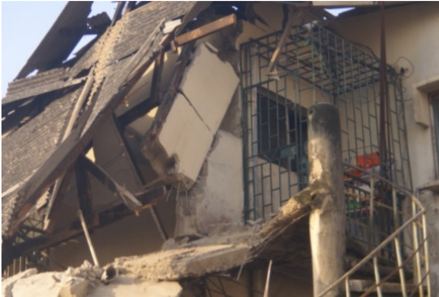
The poor state of buildings in Lagos State
