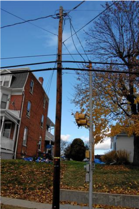
House service to Met-Ed pole Photo # 8
