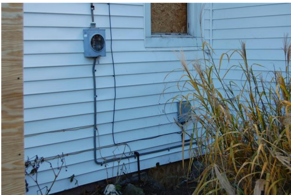
Meter base of electrical service Photo # 6
