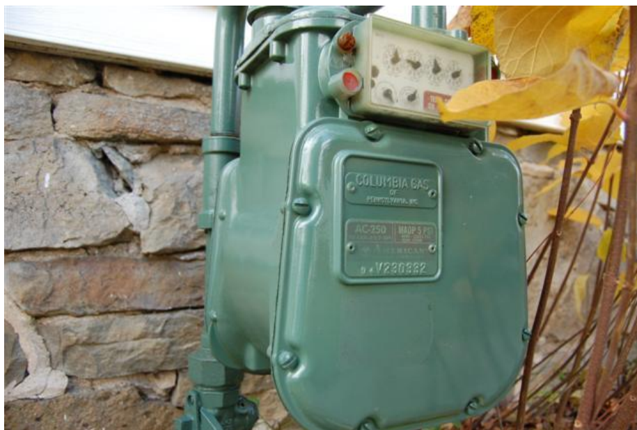
Gas meter on east side of house Photo # 15
