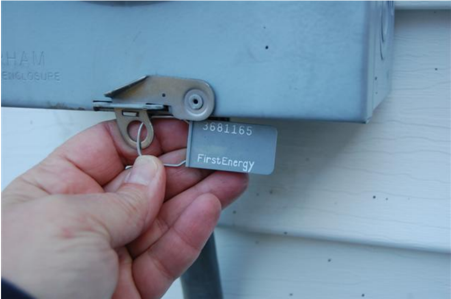
First Energy lock-out service tag Photo # 7
