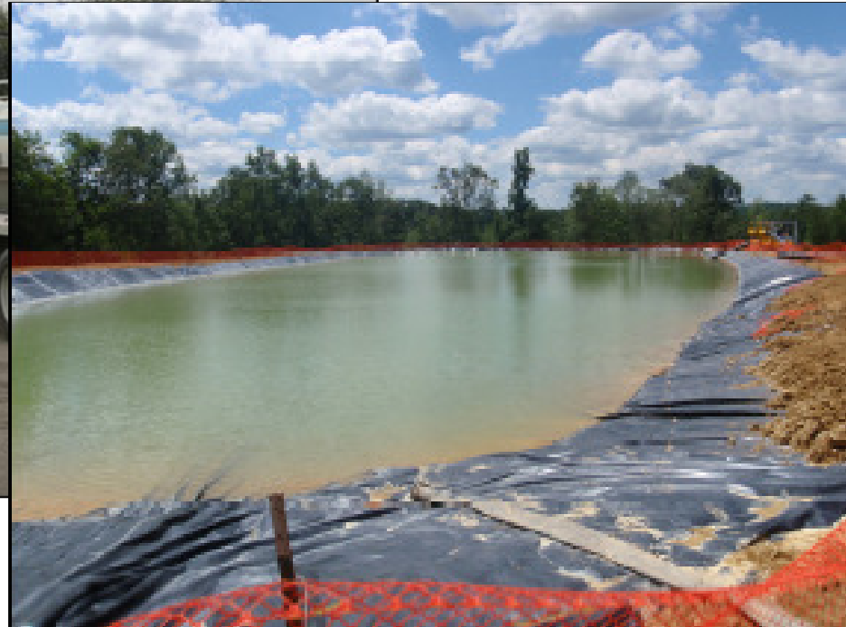
Lined Fresh Water Supply Pit from Marcellus Shale Source: DOE, Fracing Primer
